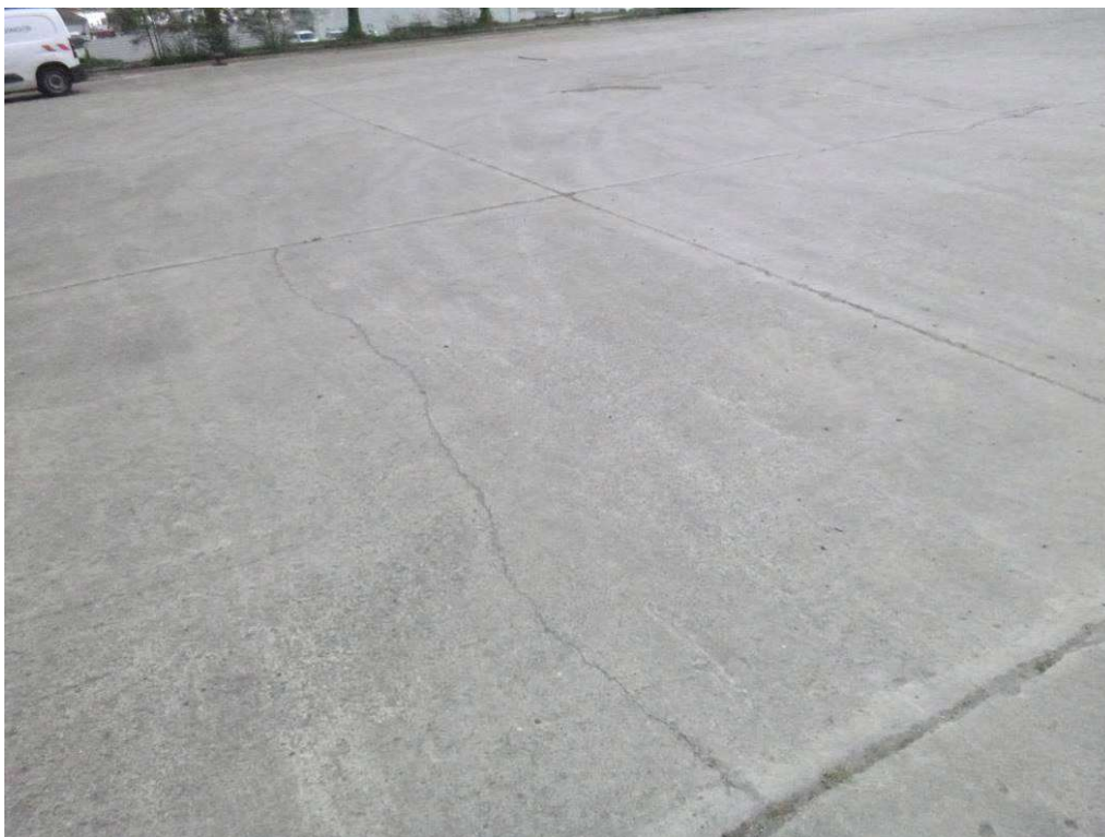
Figure 16 : Fissuration du dallage.
