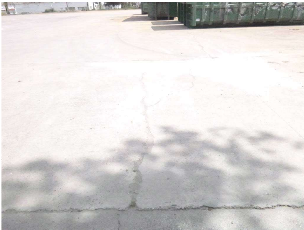
Figure 3 : Fissuration du dallage
