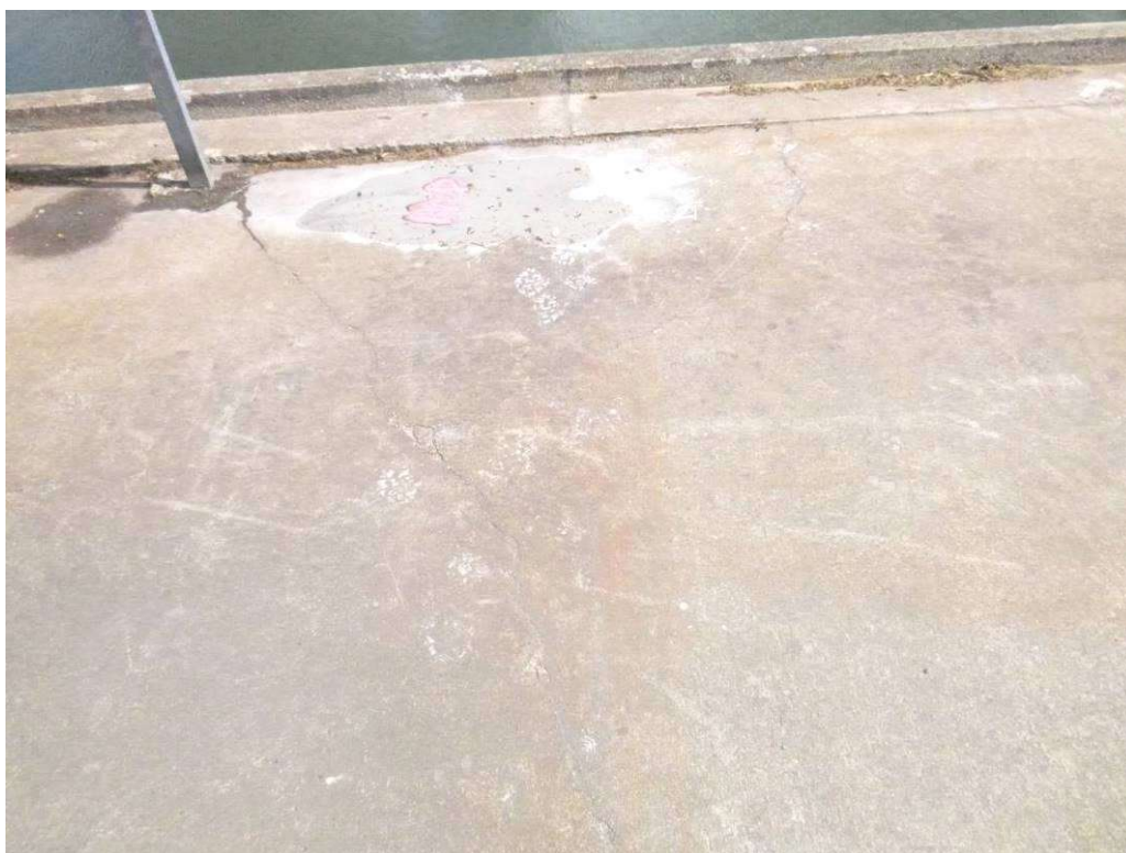
Figure 21 : Fissuration du dallage.
