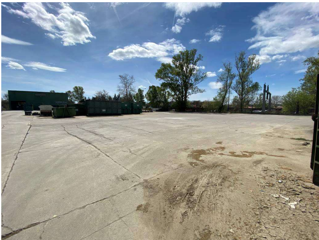
Figure 26 : fissuration du dallage.
