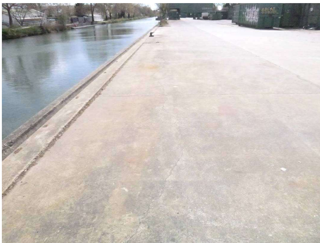
Figure 22 : Fissuration du dallage.
