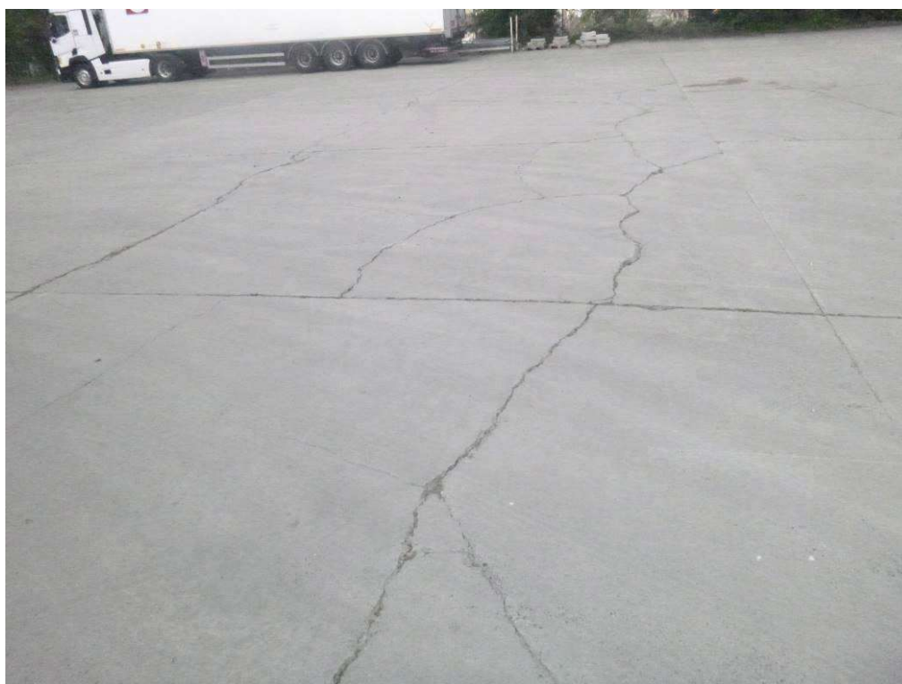
Figure 30 : Fissuration du dallage.
